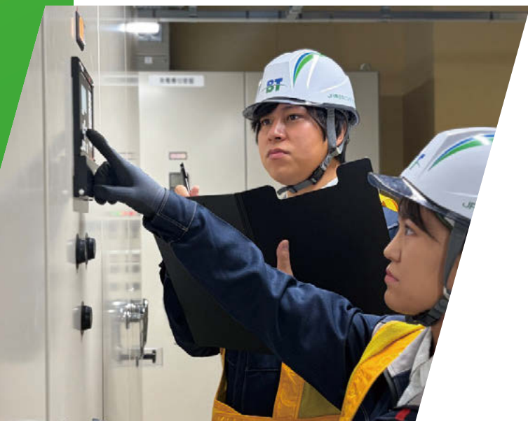
Employee engaged in switchboard inspection (JR East Facility Management Co., Ltd.)
