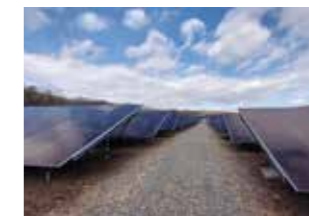
Ikeda Solar Power Plant in Tochigi Prefecture
