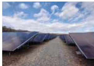
Ikeda Solar Power Plant in Tochigi Prefecture
