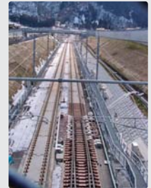
Installation of additional electric snow melters
