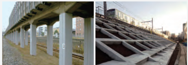
Measures for withstanding major earthquakes (seismic reinforcement of viaduct columns and embankments)
