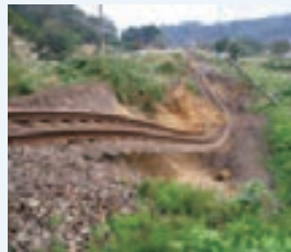
Example of damage
