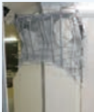
Example of damage
