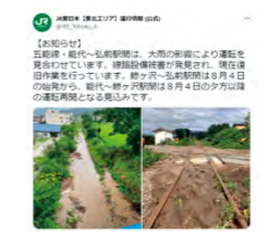
Gono Line operation suspended due to heavy rain
