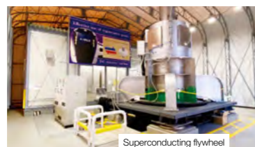
Superconducting flywheel energy storage system
