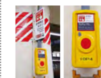
We have installed emergency stop buttons on platform pillars so that people can notify drivers, conductors, and station staff of danger.
