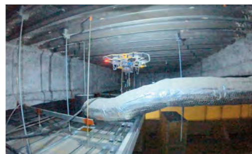
For inaccessible areas of sites, we use small drones specially designed for restricted spaces to acquire images and point cloud data.
