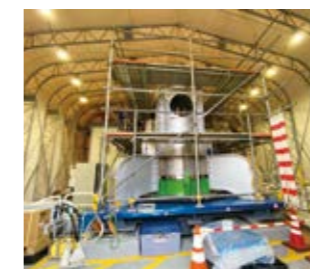
Superconducting flywheel power storage system
