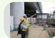
(Sendagaya) Facilities Engineering Staff member
