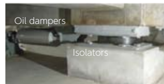
Installed vibration control system
