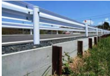
Earth retaining RC plates and damaged rails used at the road edge
