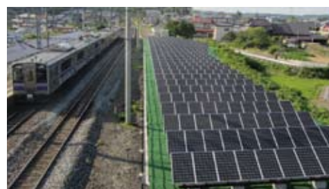
Solar panels at Hiraizumi Station
