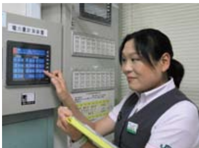
Electric energy meter facilitating employee’s activities
