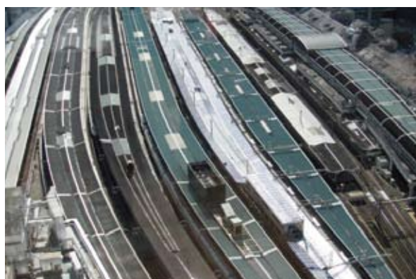
Solar panels installed atop Tokaido Line platforms (Tracks No. 9 and 10) at Tokyo station
