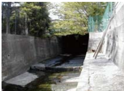
Routing tunnel groundwater to the Tachiaigawa River
