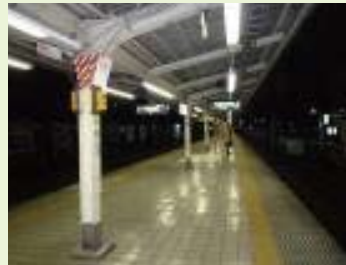
After: Intensity is even throughout the platform after changing the layout of lighting apparatus
