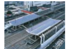
Solar panel installed atop platform roofs at Takasaki station.
