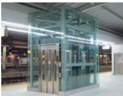
We are eliminating the need to climb steps at our stations by installing elevators and other facilities.
