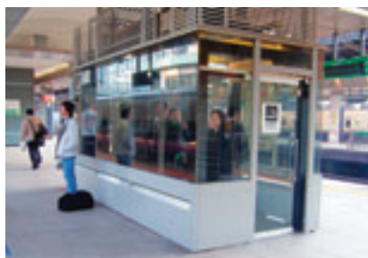
Air-purifier-equipped smoking rooms were installed on some Shinkansen platforms.
