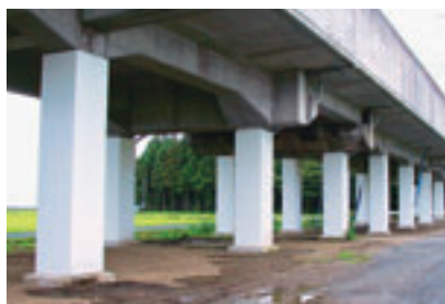
We are reinforcing seismic-resistance capabilities of elevated Shinkansen-track support columns ahead of schedule.
