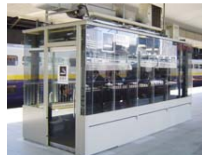
In order to promote prohibitions on smoking, completely-enclosed rooms with exhaust facilities have been installed as smoking areas on some Shinkansen platforms.
