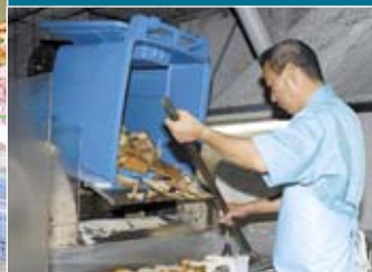
▶ Food-waste processor; about 1.5 tons of food waste is processed every day.
