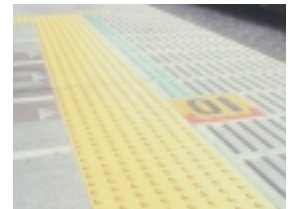
Raised tiles for guiding visually impaired persons
