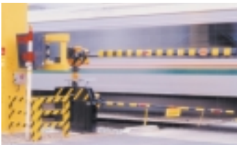
Two stage type crossing gates
