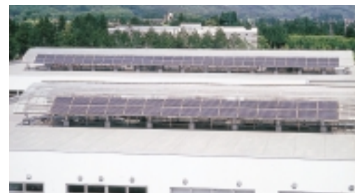
Photovoltaic generator set
