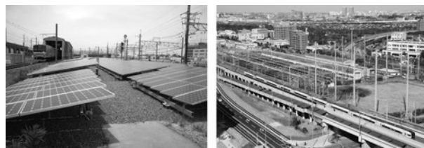
Fig. 7 PV Facilities Installed at Keiyo Rolling Stock Center
