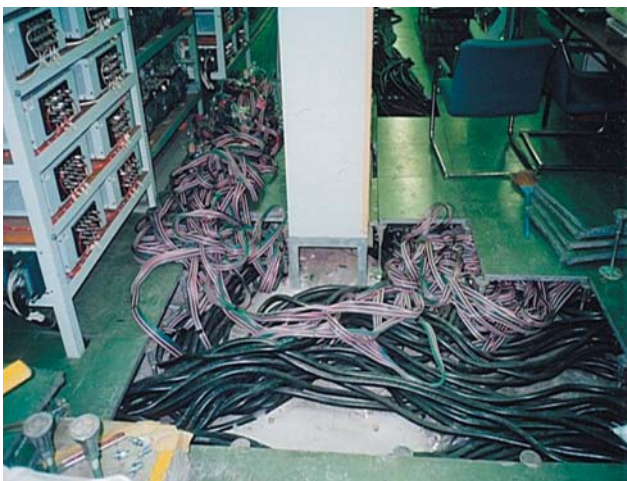
Fig. 11: Cable conditions in the current machine room
