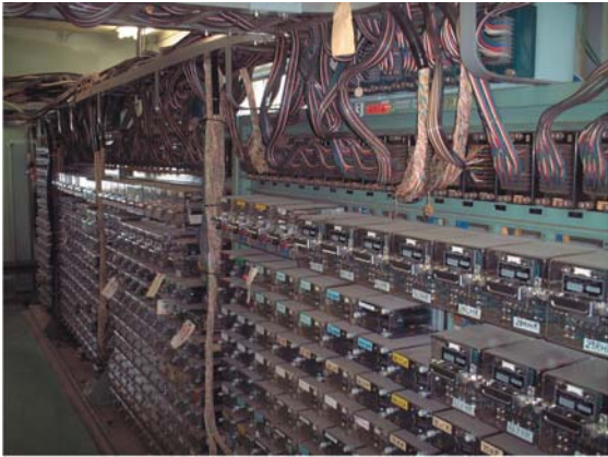
Fig.7: Relay interlocking device
