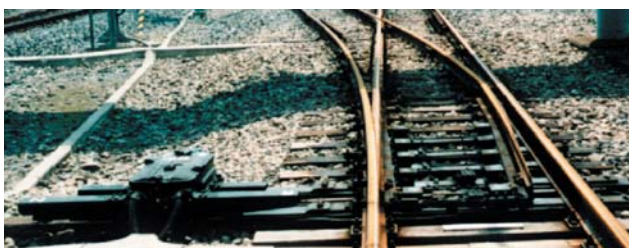
Fig.5: Switch machine (left) and turnout (right)
