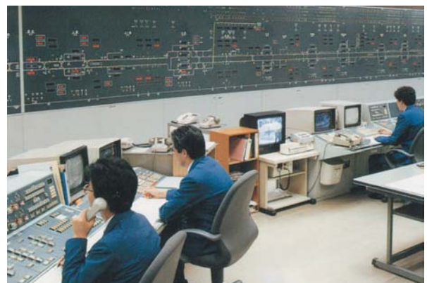
Fig.9: Dispatch center and traffic control system
