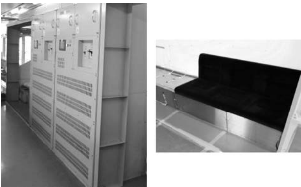
Fig. 2 Mounting of Main Circuit Battery Units (Left: Vertical setting, Right: Mounting under seats)
