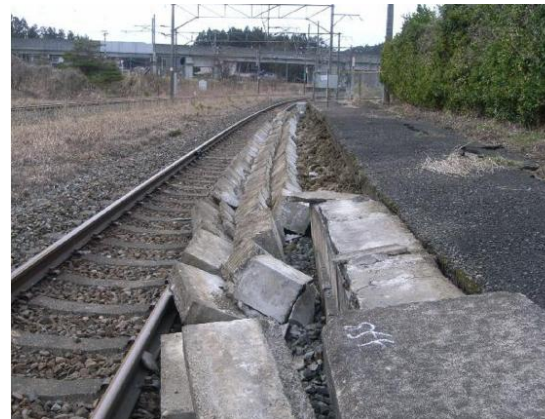
Collapse of platforms
