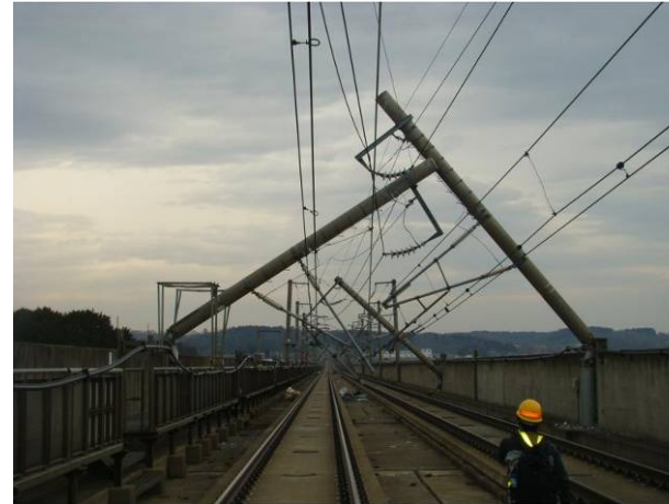
Collapse of electric poles
