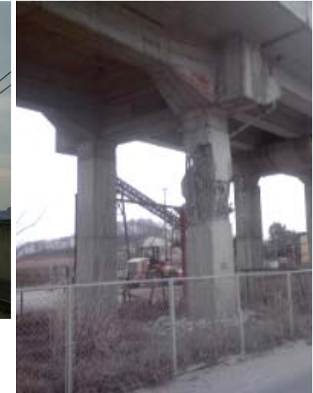
Damage to columns of viaduct
