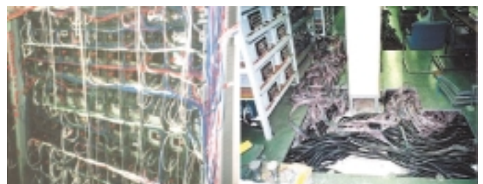
Fig. 6: Wiring and Cables in the Existing Signal Equipment Room
