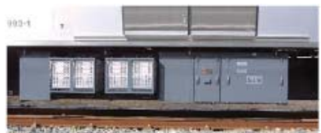
Fig.10: Auxiliary Power Source Equipment with Functions for Self Diagnosis and Emergency Measures
